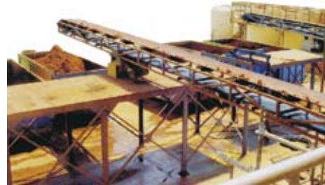
Sludge management system at the outlet of water treatment plants.
