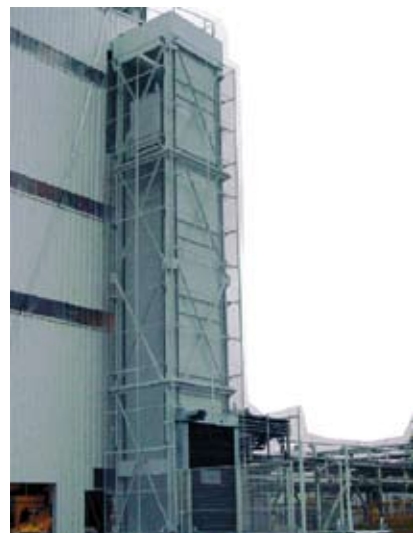
Pallet elevator to 16 metres.
